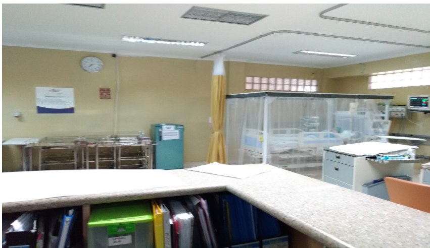
Picture 1: Portable HEPA Filter in ICU Room
